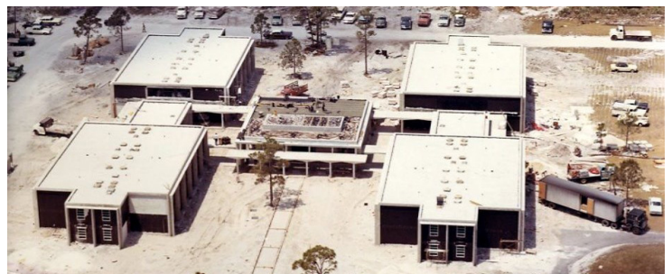
Above: Construction of South Dorm (Patton Hall, deHoernle Residential Center) in 1967. Photo/Lynn University Archives.
