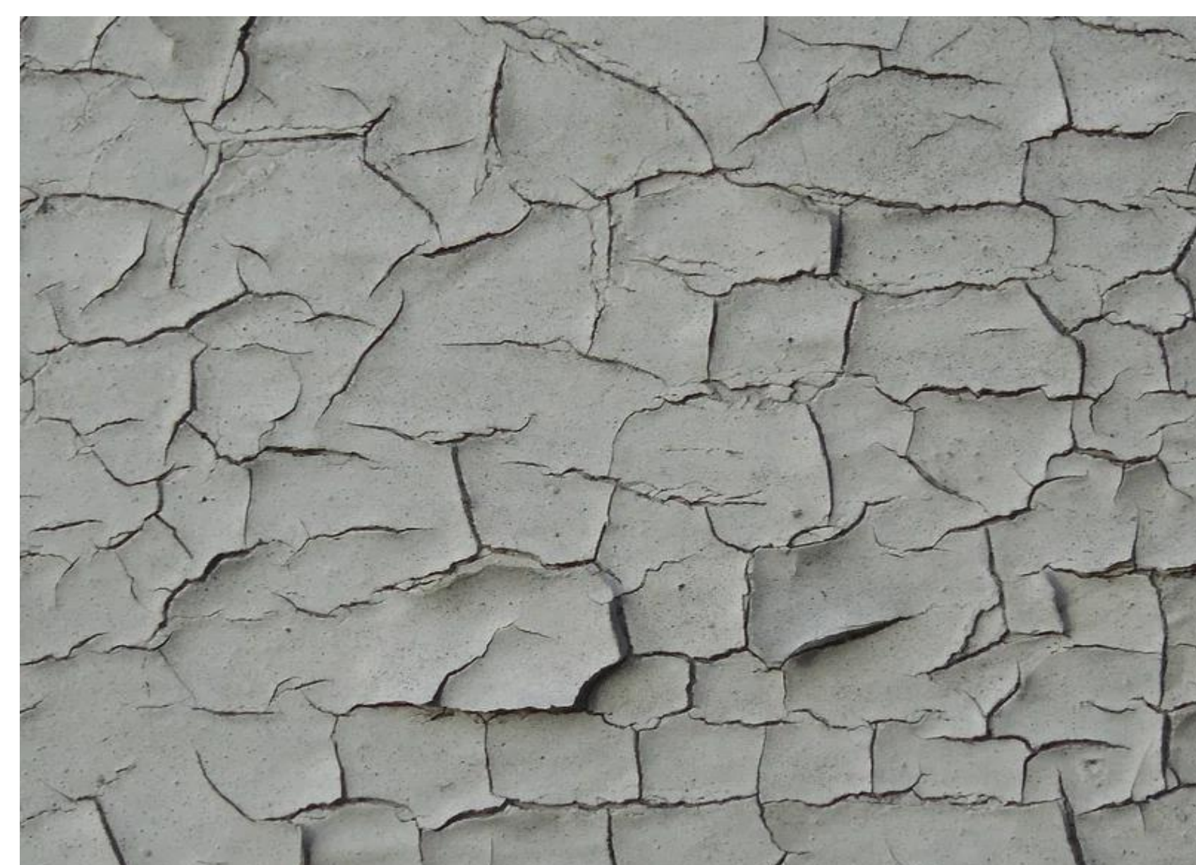
Fig 1. Chipping paint at scene.
